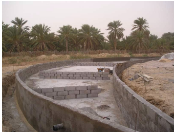
Figure 8b. Baffle walls to ensure sewage water’s proper residence time and avoid short-circuiting.
