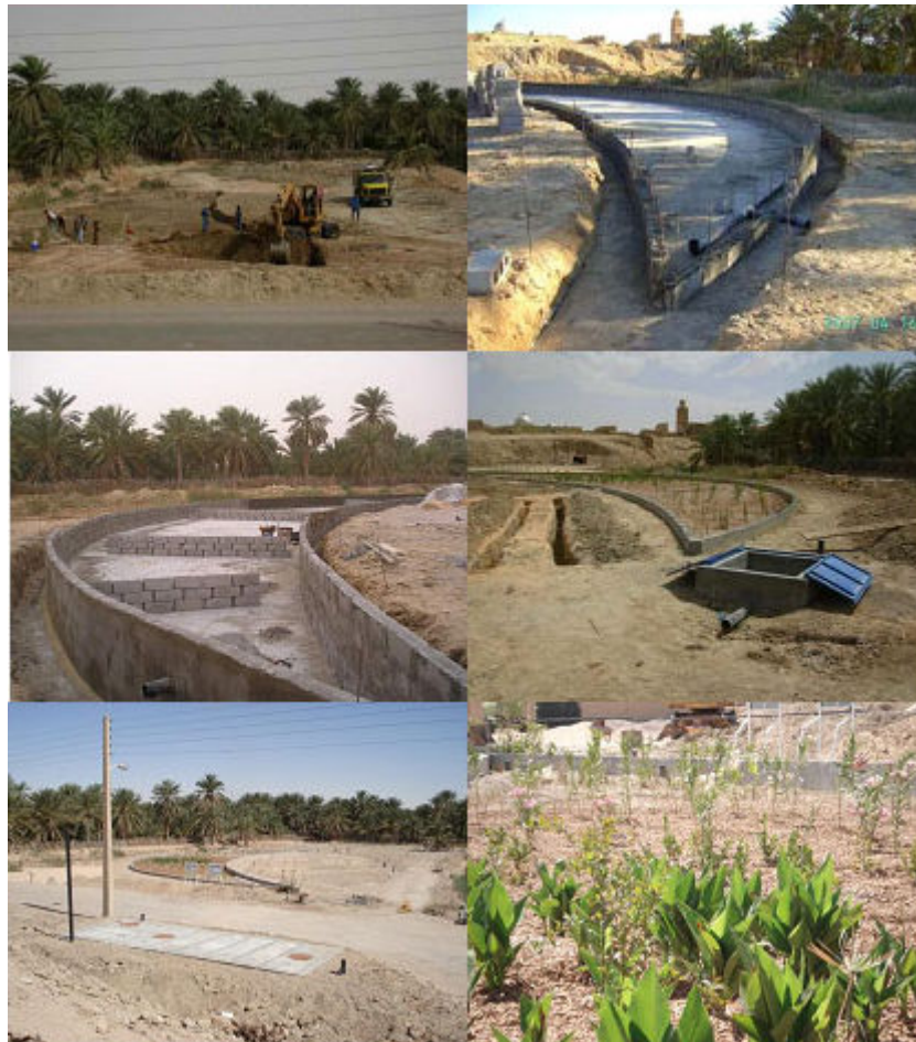
Figure 8a. Several stages of the construction of the Wastewater Gardens at Temacine, Algeria. Top right: excavation begins of the basin; top left; after the concrete floor slab is poured, concrete blocks with steel reinforcing make the side walls; Middle right: walls are plastered and baffles made inside the basin to make water flow more slowly through the system; middle left: control box with airtight lid is installed and subsoil irrigation, leachdrain trenches begun. Bottom right: view from the old Ksar of 37.5\text{m}^3 septic tank (foreground), planted WWG and leach drains. Bottom left: closer view of WWG plants a few months after planting.
